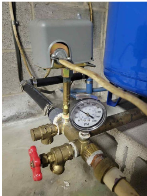
Well switch and pressure gauge
