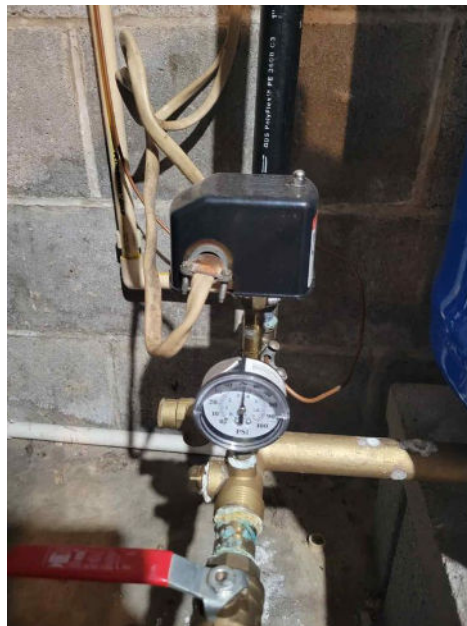
Well switch and pressure gauge
