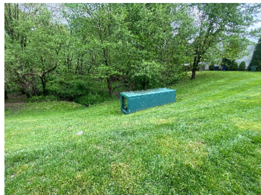
Detention pond and catch basin
