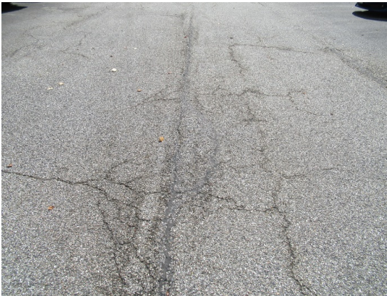
Diggers Lane cracks
