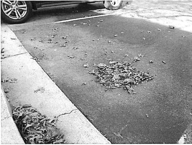
Pavement settlement at Hunt Hill Drive
