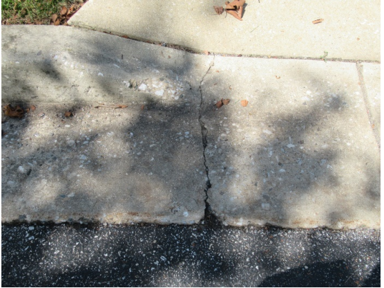
Curb and gutter crack
