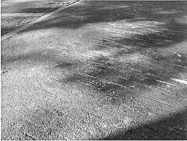
Abraded pavement near speed hump on Steepridge Drive
