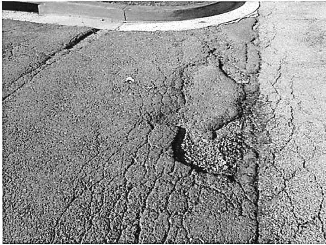
Alligator cracks, pothole and settled pavement at Critter Court
