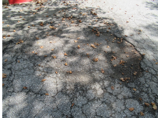
Diggers Lane cracks and pavement deterioration
