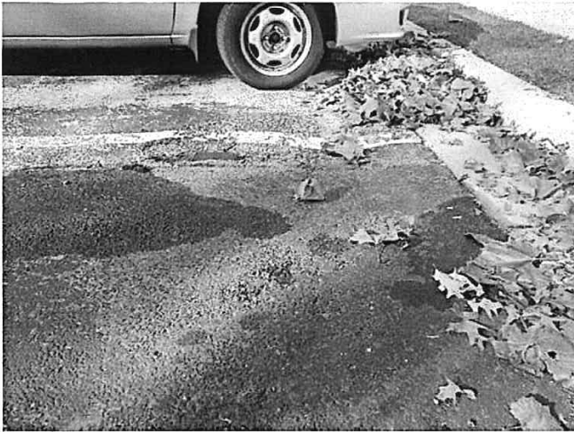
Pavement settlement at Chipwood Court
