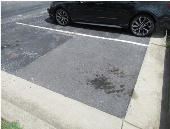
Whisper Way patching and vehicular fluid stains
