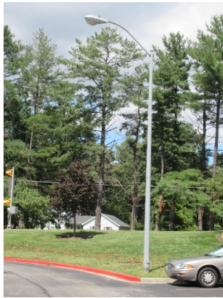
Light pole and fixture
