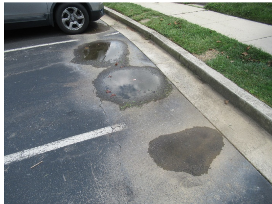
Hunt Hill Drive pavement ruts
