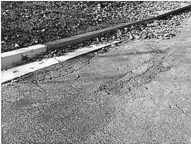
Pavement settlement and patch at Chipwood Court
