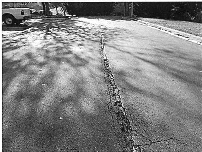
Centerline cracks at Hunt Hill Drive
