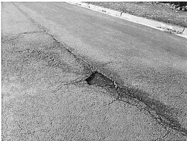
Failed pavement at Critter Court
