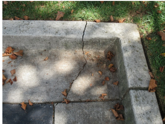
Curb and gutter crack
