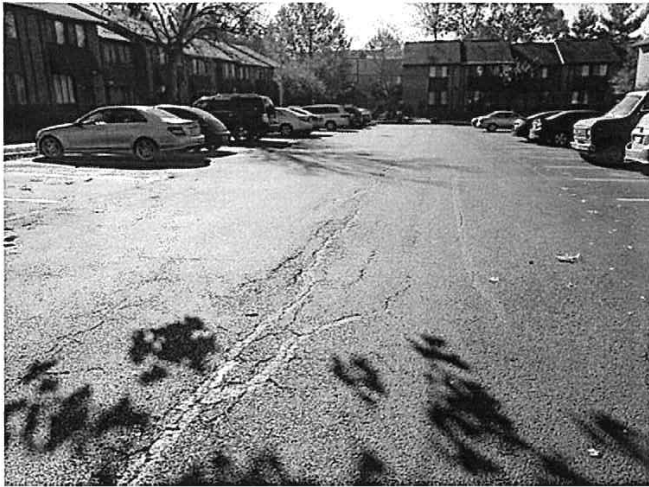
Cracks and previous crack repairs at Whisper Way pavement
