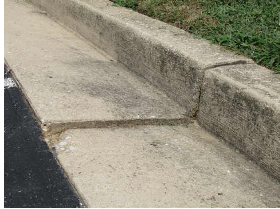
Curb and gutter settlement
