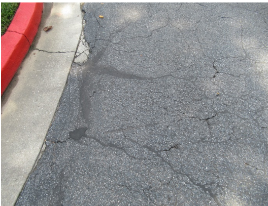
Hunt Hill Drive cracks
