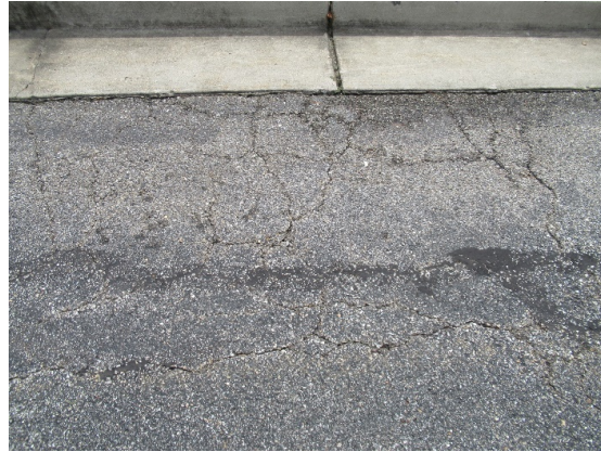
Chipwood Court Cracks
