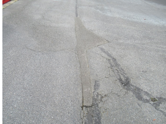
Critter Court centerline patching and cracks
