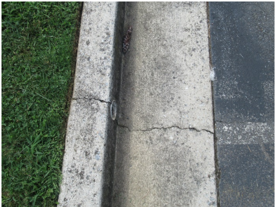
Curb and gutter crack
