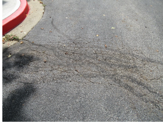
Steepridge Court cracks
