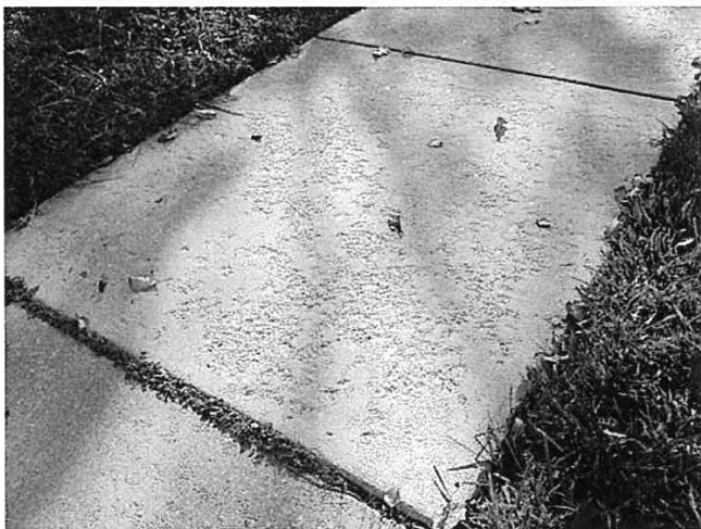
Spalled concrete sidewalk
