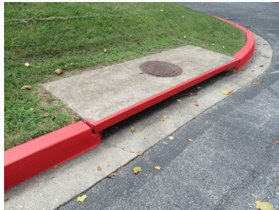
Catch basin overview; we note minor cracks at the concrete gutters adjacent to the catch basin indicating possible minor settlement
