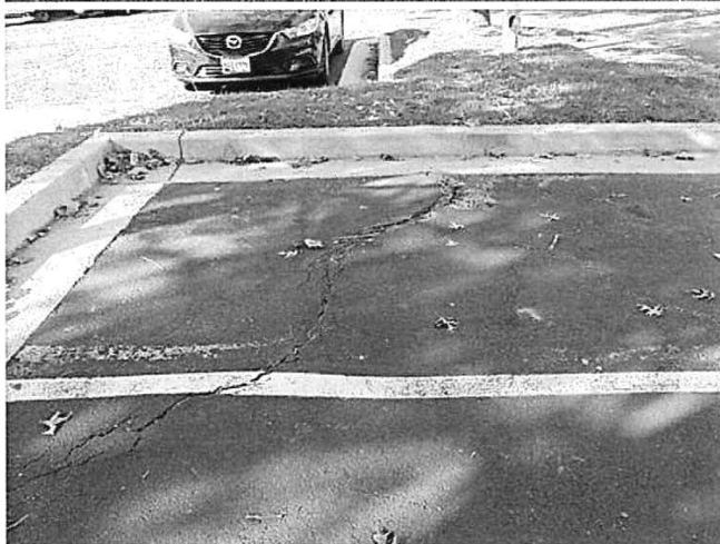
Pavement movement likely due to tree roots on Whisper Way
