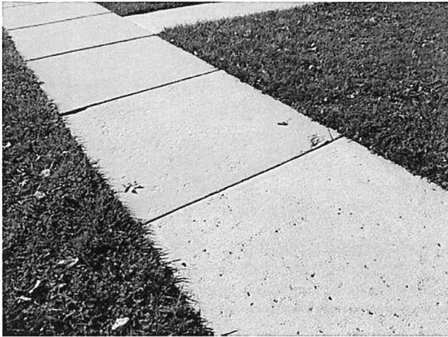
Spalled concrete sidewalk
