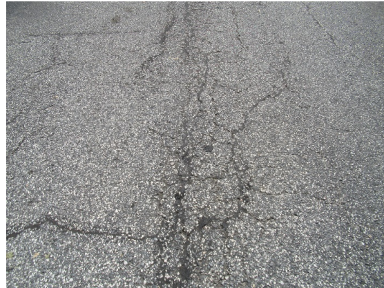
Whisper Way cracks
