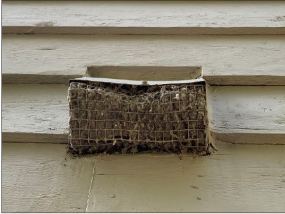
Photo 13: Example of an exterior vent which should be cleaned as part of regular annual maintenance.
