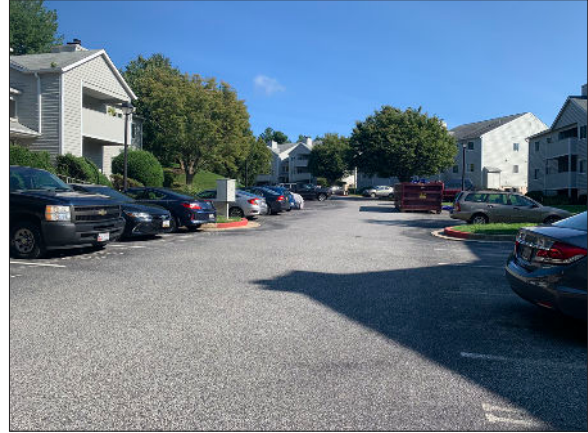
Photo 2: Asphalt conditions near building 2211 & 2212.
