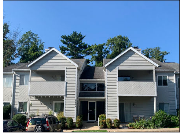
Photo 10: Typical example of common area doors and windows, as well as exterior conditions of building 2218.
