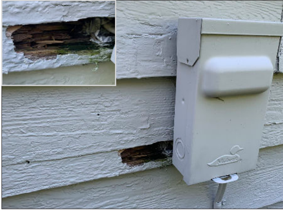
Photo 9: Example of siding repairs needed on building 2218.
