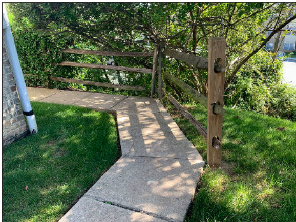
Photo 7: Split rail fence at the rear of building 2215. Note the branches above the corner are protruding over the walkway and should be removed as soon as possible.
