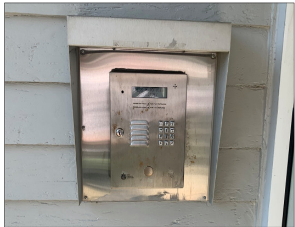
Photo 16: Example of the entry system in each building.
