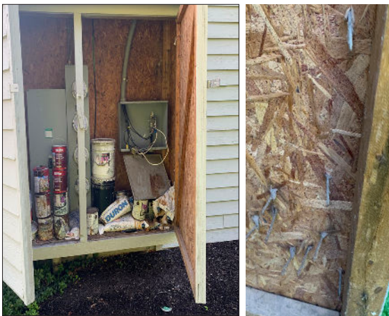
Photo 11: Utility room located on the northern side of building 2218. Note the nails on the inside of the utility room doors.
