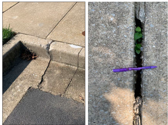
Photo 4: Example of curb and sidewalk repairs as noted in our report near building 2218 and 2215.
