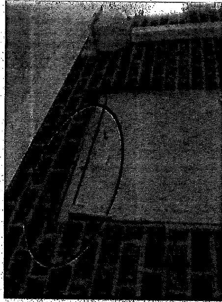
Photo 15: Exterior metal door on the roof was in poor condition and should be scheduled for replacement.
