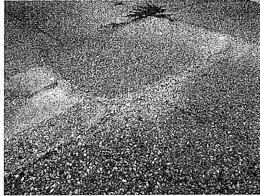
Concrete at plaza deterioration and cracks
