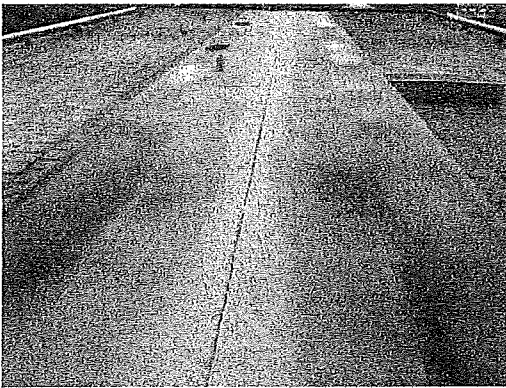
Modified bitumen roof section – Note: wear
