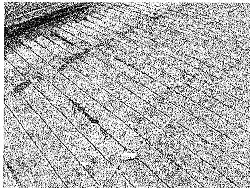
Concrete driveway cracks and deterioration
