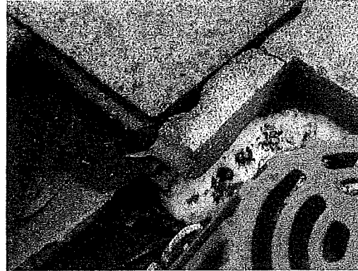
Inverted roof deterioration
