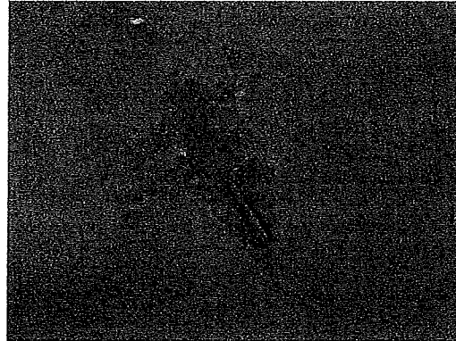
Concrete spall and exposed rebar
