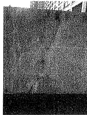
Retaining wall cracks
