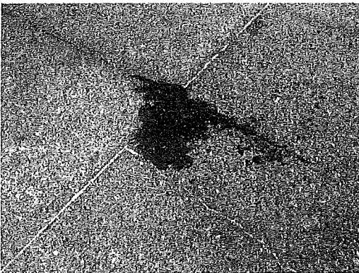
Concrete at plaza deterioration and cracks
