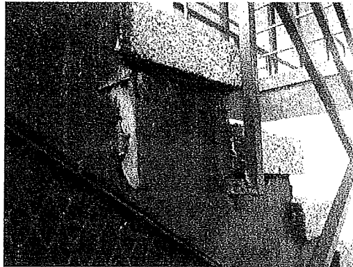
Metal paint finish deterioration and rust
