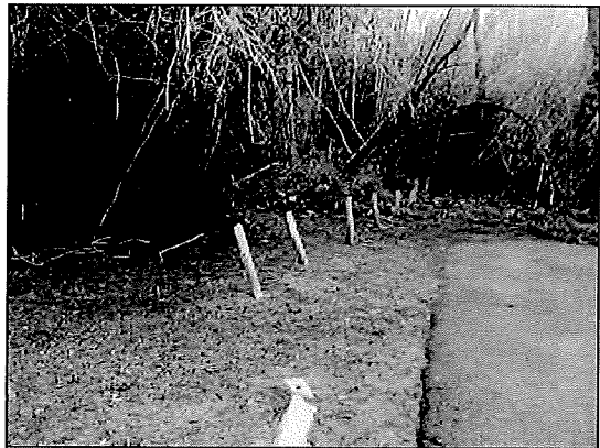
Photo #14. Damaged bollards, 5601.
