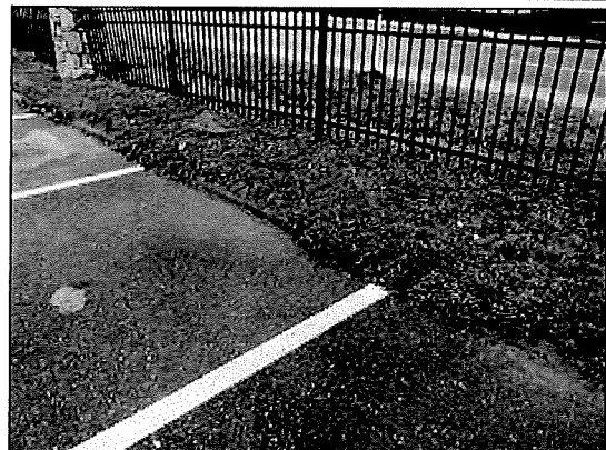
Photo #4. Asphalt curbs appear not to have been renewed in conjunction with the previous paving project and are no longer effective.
