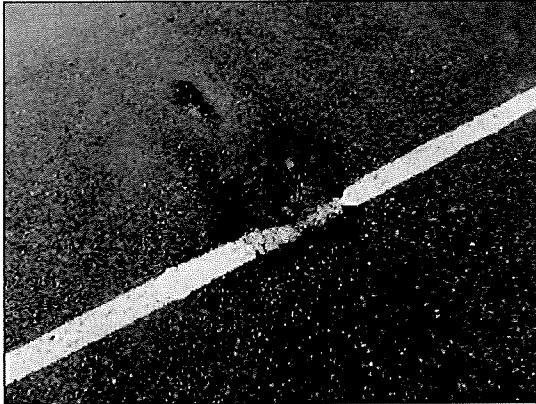
Photo #7. Typical damaged asphalt pavement.
