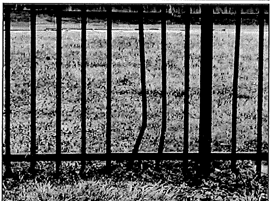
Photo #18. Typical damaged metal fence.
