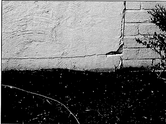
Photo #51. Typical defect in the Pool Building masonry façade.
