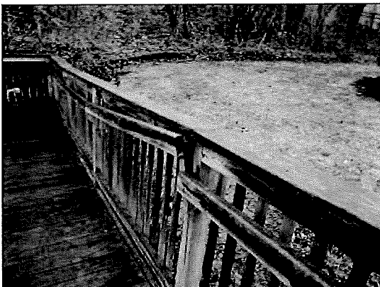
Photo #33. Defects in the railings at the swimming pool facilities are a hazard.
