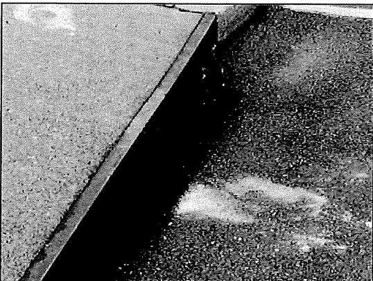
Photo #17. Pavement installations have reduced the opening into the drop inlet.
