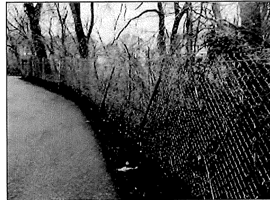
Photo #12. Damaged perimeter chain link fence near 5601.
