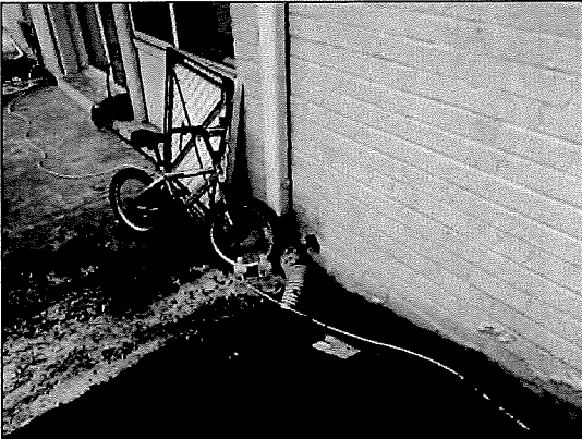
Photo #19. Typical defective grading at building.
