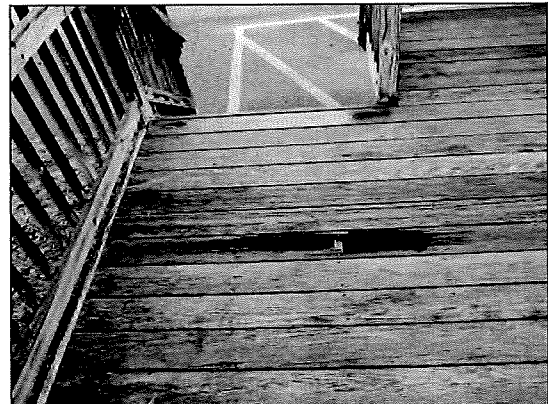
Photo #22. Defects in the deck and ramp at the swimming pool facilities are a hazard.
