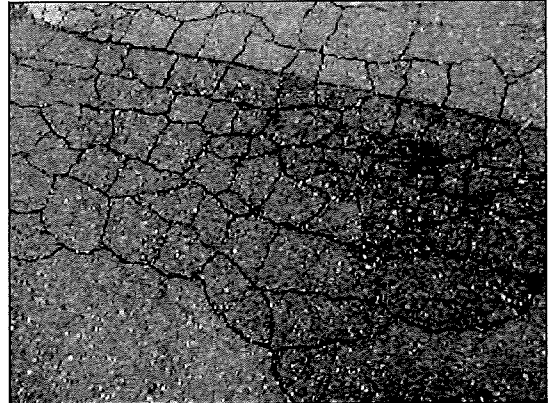
Photo #20. Typical severely alligatored asphalt pavement.
