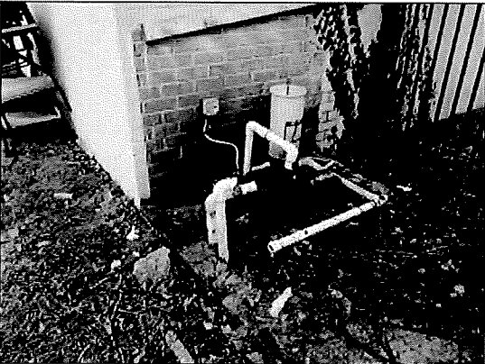
Photo #27. Unused equipment adjacent to the Pool Building has not been properly abandoned.
