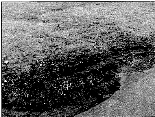
Photo #9. The lack of a curb and defective grading adjacent to the asphalt pavement will reduce the economic life of the pavement.
