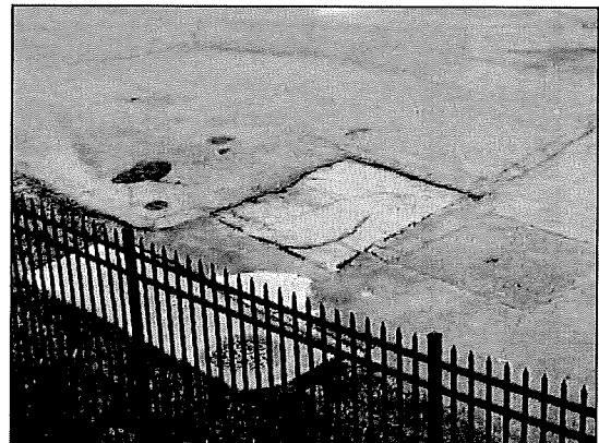
Photo #54. Defective asphalt pavement.
