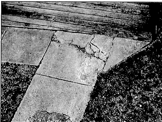
Photo #53. Sidewalk defects are a potential trip hazard.
