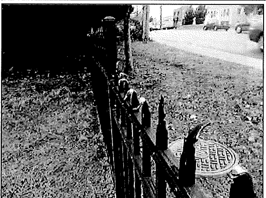
Photo #42. Damaged decorative fence along Chillum Road.
