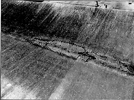
Photo #49. Precast concrete roof structure is not pitched to discharge water.
