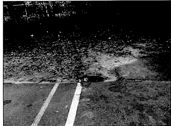
Photo #8. The lack of a curb and defective grading adjacent to the asphalt pavement will reduce the economic life of the pavement.
