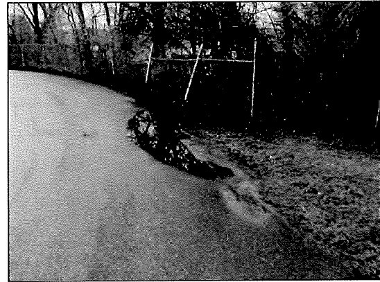
Photo #10. Defective grading adjacent to the asphalt pavement impounds water and will cause accelerated deterioration.
