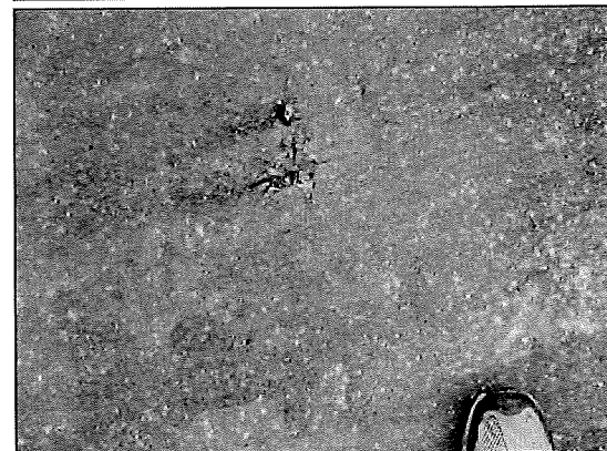
Photo #48. Defects in the precast concrete roof structure impound water and will result in accelerated deterioration.
