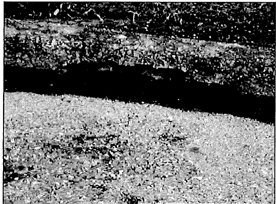
Photo #38. Typical deteriorated wheel stop (near 5601).
