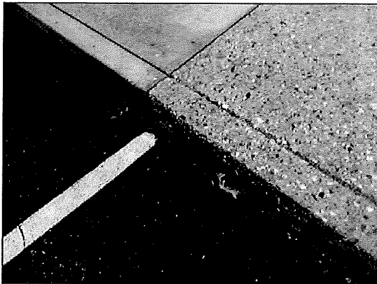
Photo #15. Defective pavement installation impounds water between the pavement and the curb.
