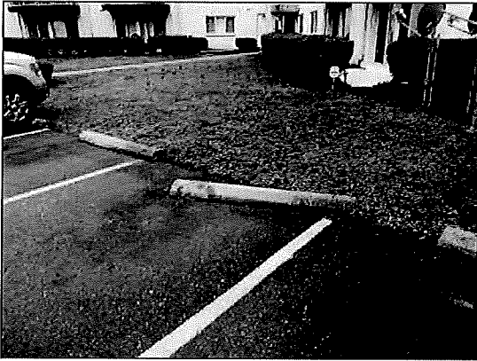
Photo #13. Improperly installed wheel stops, 5601.
