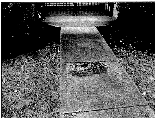
Photo #35. Typical sidewalk defect that is a potential trip hazard.
