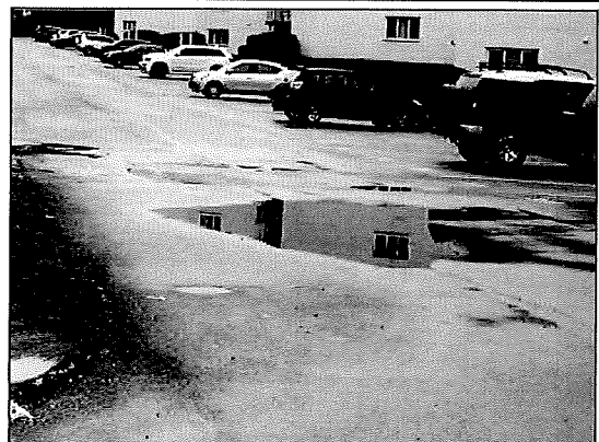
Photo #6. Typical standing water on the asphalt pavement.
